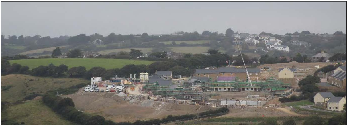
Looking north west with TL30A in the foreground
